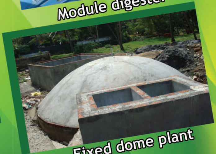
Institutional biogas plant
